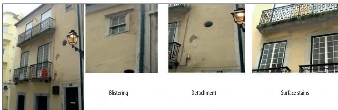
Fig. 2. Case study representative of the end of the service life of façade paintings (degradation severity around 20%)
